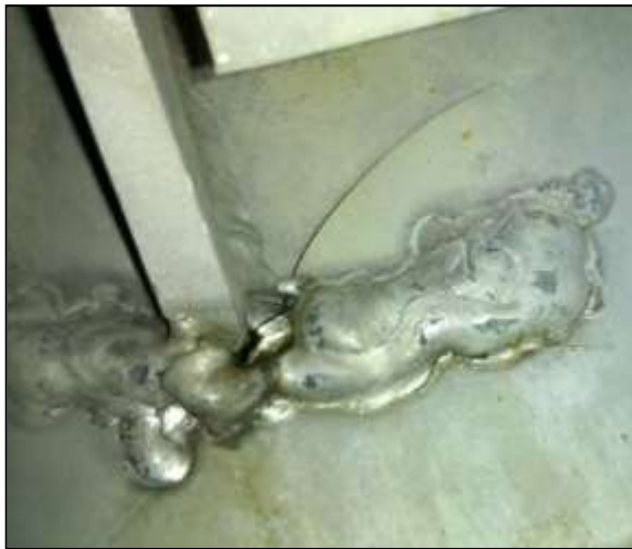
Figure 12: Fatigue Cracking in the Vibratory Conveyor's Support Structure, Partly Covered By Repair Weld
