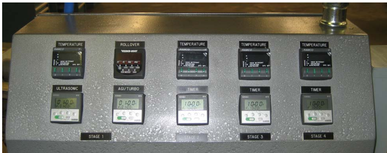
Main Control Panel Timers and Controllers
