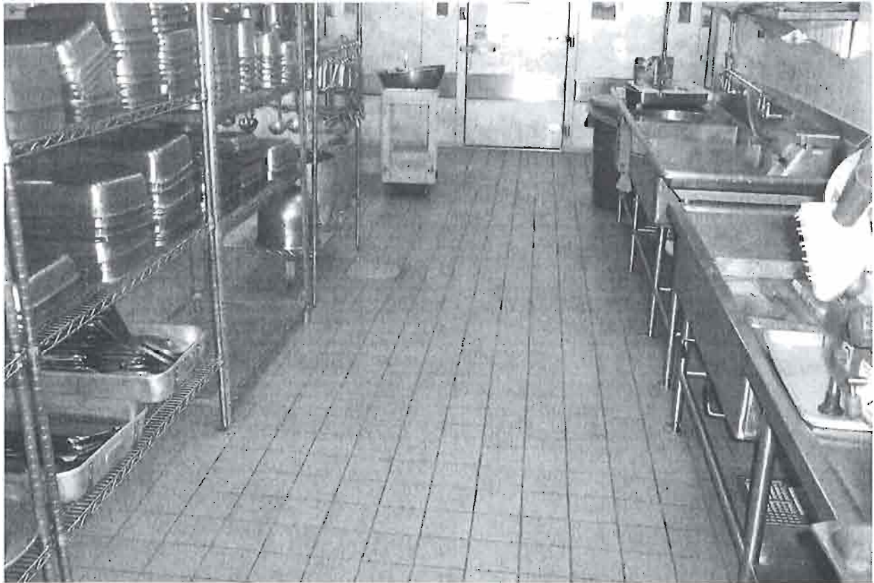
Photo of floor without slip and wet surface sign.
